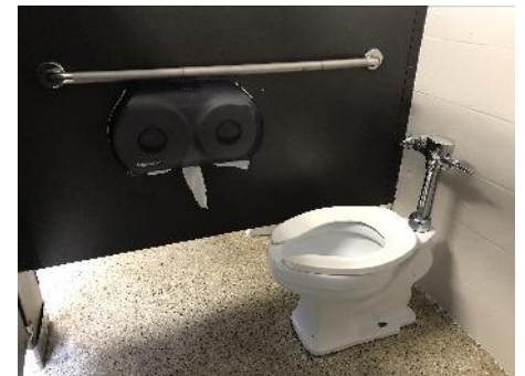
Centennial Arena, Toilet, Requires Back Support & L Grab Bar
