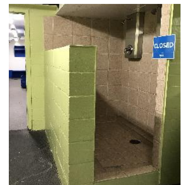
Centennial Arena, No Accessible Showers
