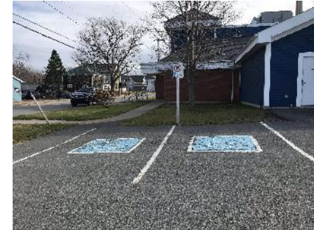
Police Station, Accessible Parking, No access lane for driver & passengers
