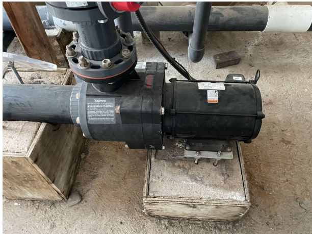
Figure 7 Existing Pool Filter Pump
