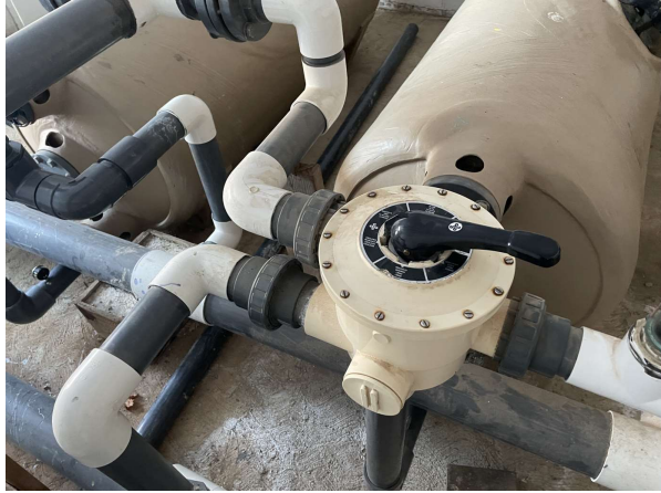
Figure 8 Existing Sand Filters
