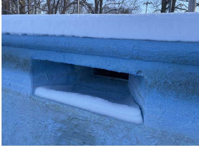
Figure 5 Existing Skimmer Openings, No Grilles
