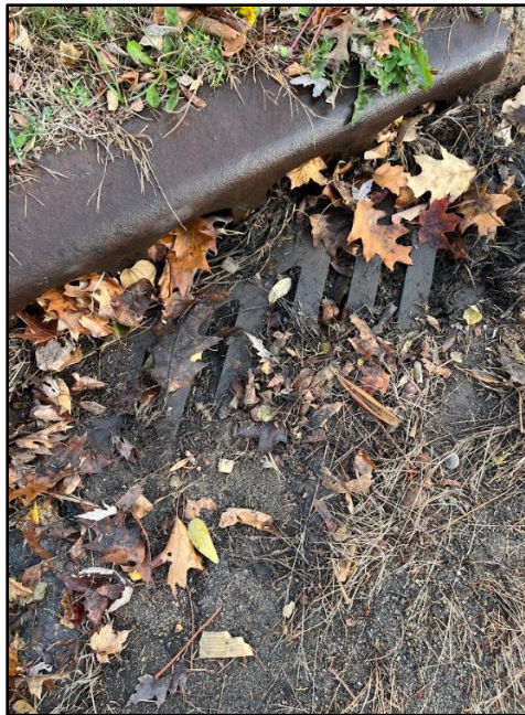
Figure 3-4: Reduced Capacity Catch Basin on Main Street (November 6, 2024)
