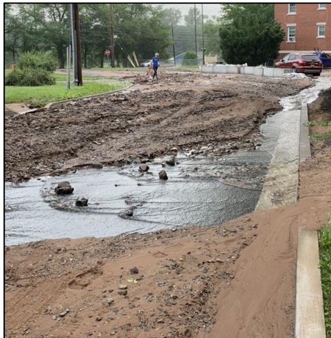
Figure 3-3: Sediment and Bank Material Deposited on Condon Avenue Following the July 11, 2024, Rainfall Event (Photo Provided by a Resident of Condon Avenue)
