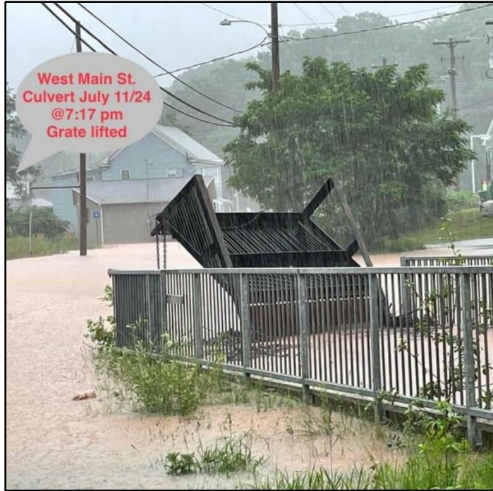
Figure 2-2: Culvert Located at Intersection of West Main Street and Harvest Moon Trail Ditch on July 11, 2024 (Photo Provided by Kentville Resident)
